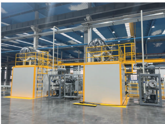
Vacuum Oil Injection Line >>>
