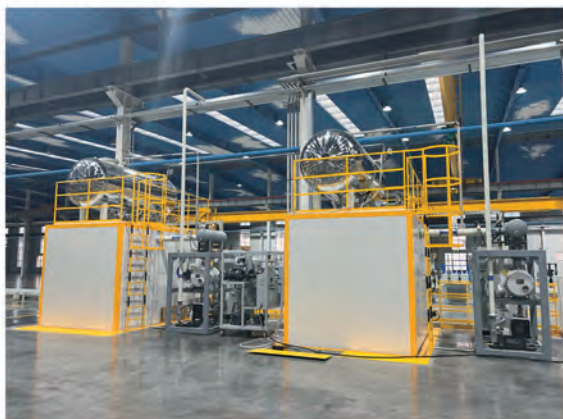
Vacuum Oil Injection Line >>>
