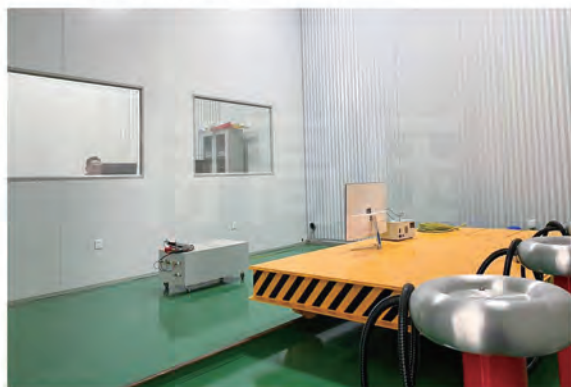
Partial Discharge Laboratory >>>
